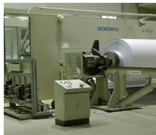
The paper finishing area
